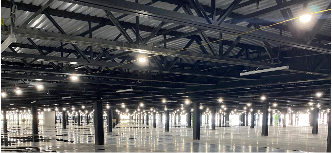
EPCO's LED CordLights illuminating a construction site after the exterior has been enclosed.
